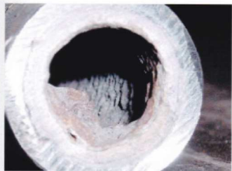
Before installing ISB ( Scale in pipe )
