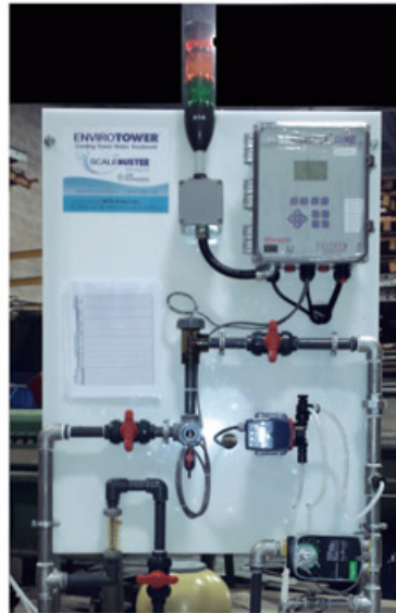
Control Skid Front View
